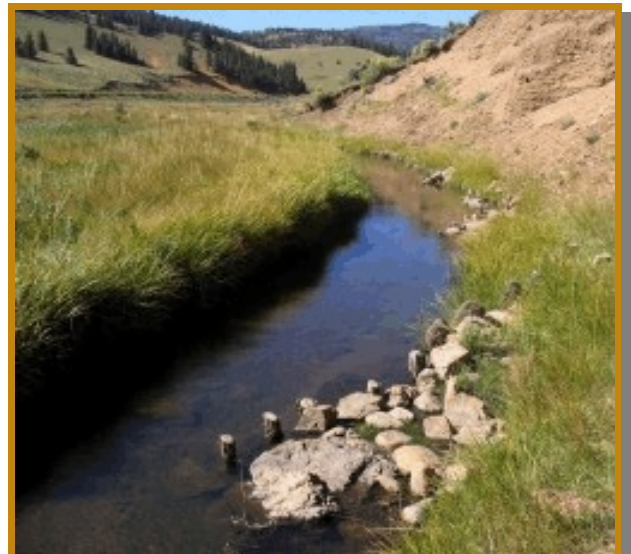
Post vanes installed along Comanche Creek -- note sedges and grasses re-establishing along raw right bank.
